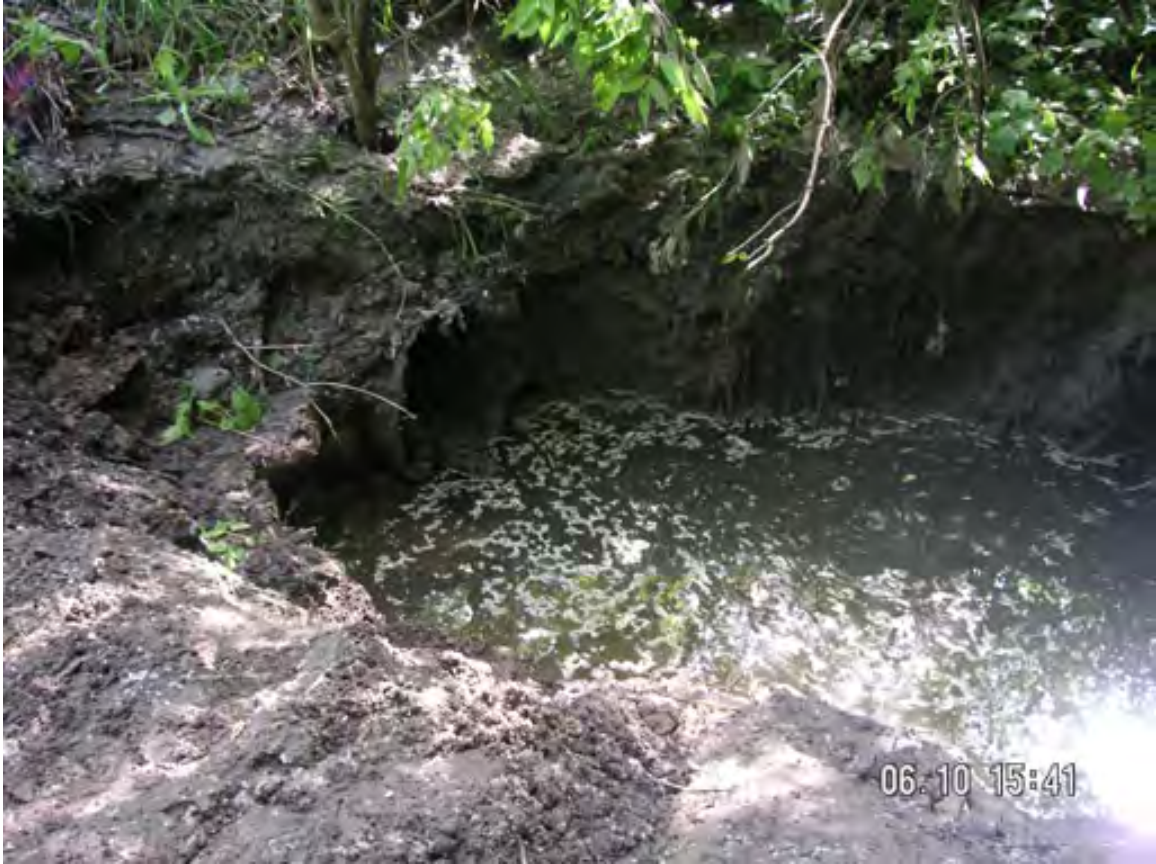
Figure 2. - The driveway culvert inlet, buried in silt.
